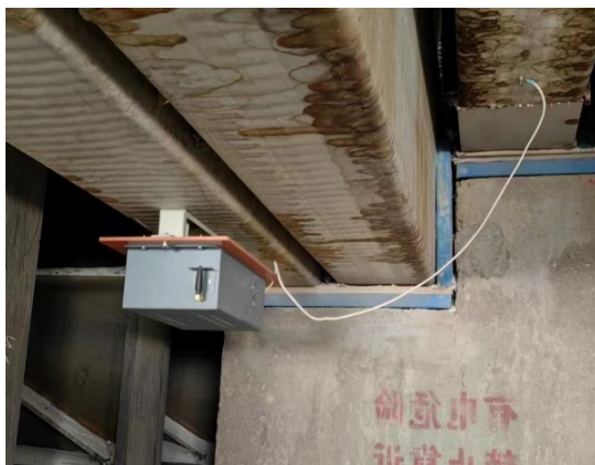
Figure 5. Cell bypass shunt data collection module.
